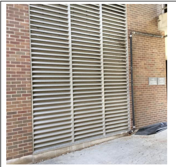
Air intake louver (close view)
