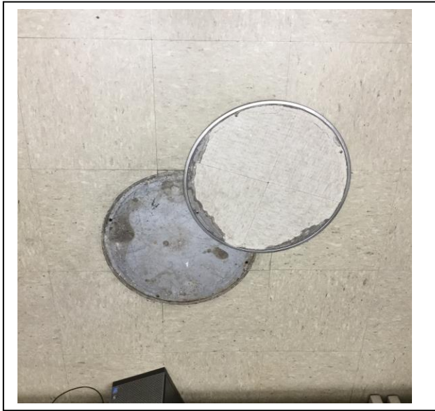
Cable bank – for cable storage
