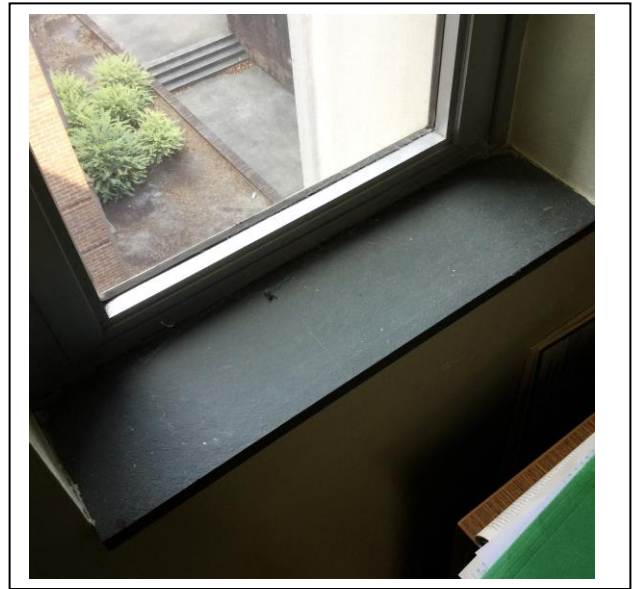
Debris and stain on window
