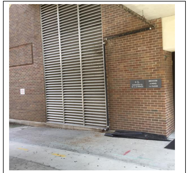
Air intake louver
