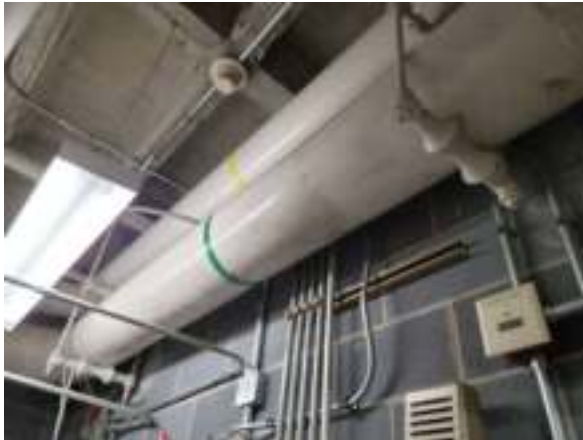
Photo #27 Non-asbestos containing white canvas wrap on 12"-14" pipes with asbestos-containing black mastic and OSHA-regulated (<1% asbestos) hard TSI elbows/joints (HA #21 and 22)
