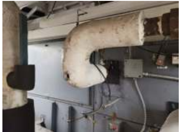
Photo #10 OSHA-regulated (<1% asbestos-containing) hard TSI elbows/joints with non-asbestos containing canvas wrap 6"-8" (HA #6)
