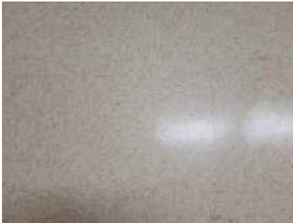
Photo #23 Asbestos-containing black floor mastic under non-asbestos containing 12" x 12" white with tan specks floor tile (HA #17)
