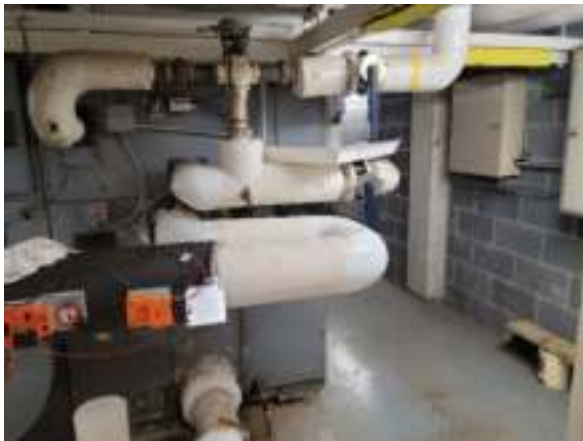
Photo #3 Typical view of mechanical room.
