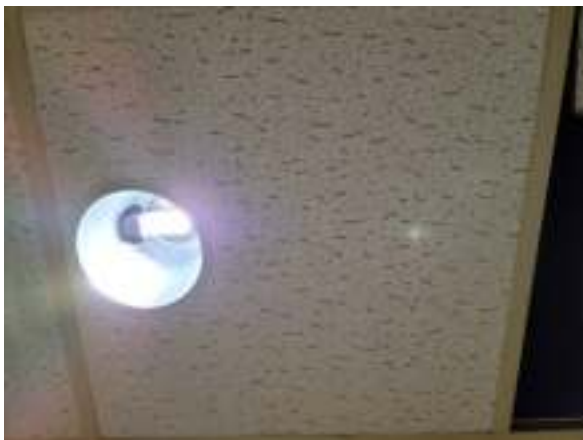
Photo #25 Non-asbestos containing 2' x 2' white ceiling tile with dots and fissures (HA #19)
