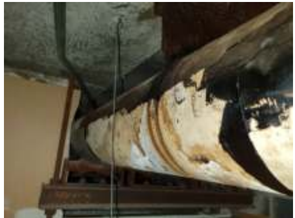
Photo #30 Asbestos-containing black mastic on fiberglass pipe insulation (HA #26)
