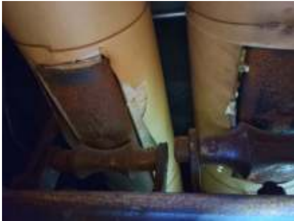
Photo #33 Non-asbestos containing brown paper over brown pipe insulation (HA #29)
