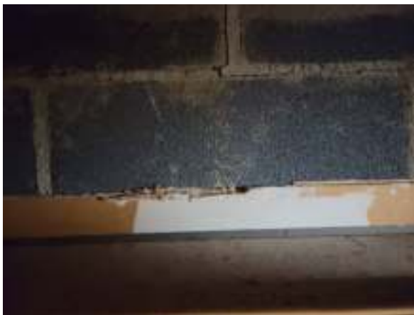
Photo #5 OSHA-regulated (<1% asbestos-containing) drywall and joint compound (HA #1)
