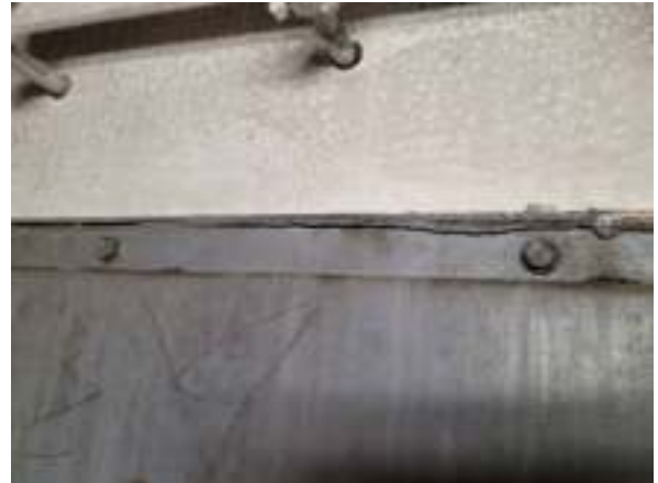
Photo #22 Asbestos-containing black seam caulk at AHU/Duct Joint (HA #16)
