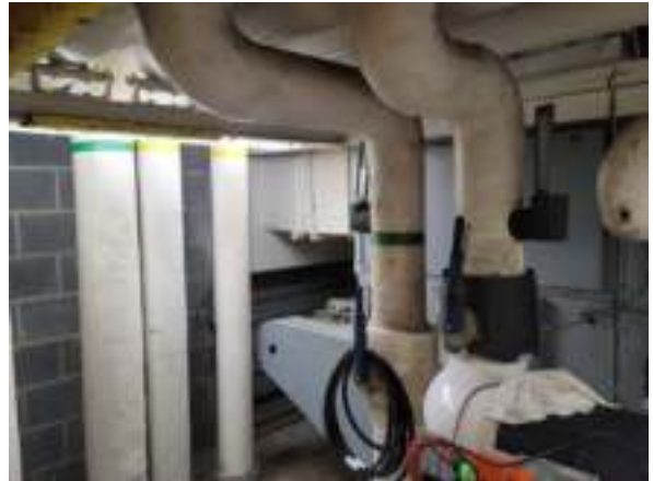
Photo #8 Non-asbestos containing white canvas wrap on 6"-8" pipes with asbestos-containing black mastic (HA #4)
