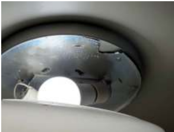
Photo #29 Asbestos-containing gray foil-backed light insulation (HA #25)
