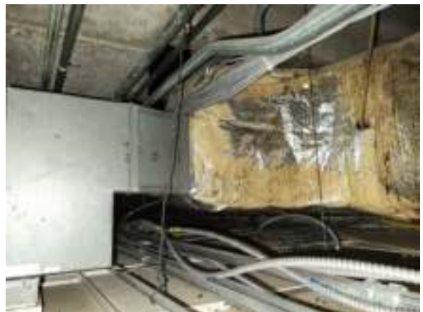
Photo #32 Non-asbestos containing yellow HVAC fiberglass duct insulation glue (HA #28)
