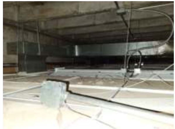
Photo #4 Typical view of plenum on 1 st through 3 rd floors.
