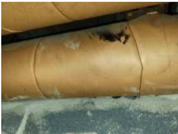
Photo #31 Non-asbestos containing brown paper and white canvas over fiberglass pipe insulation with asbestos-containing black mastic (HA #27)
