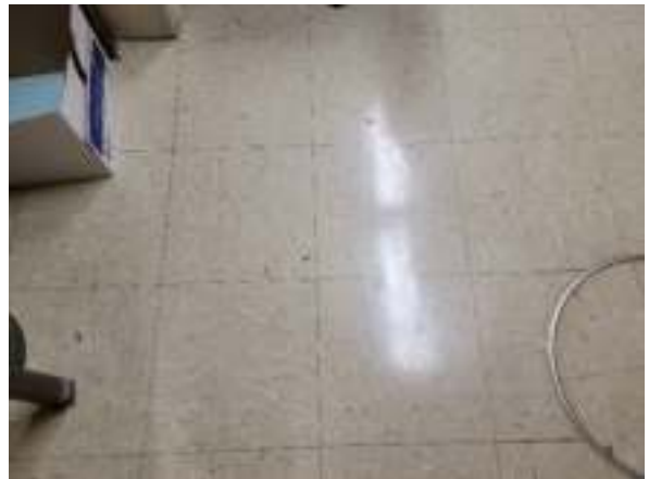
Photo #16 Asbestos-containing 12" x 12" gray with brown and black specks floor tile and mastic (HA #12)
