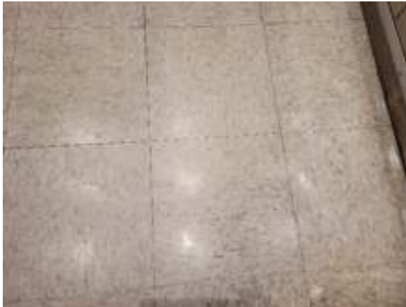
Photo #21 Non-asbestos containing 12" x 12" tri-gray floor tile and mastic (HA #15)
